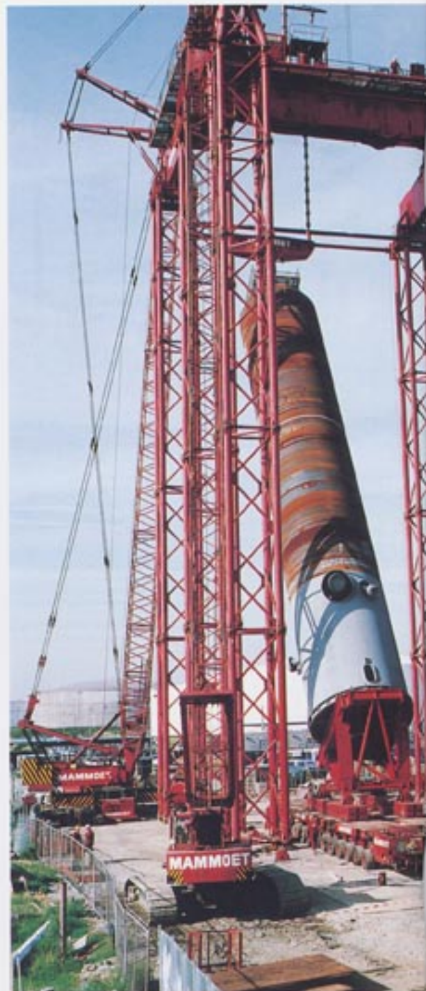
Mammoet's Hydra-Jack system: a professional and reliable lifting solution in a confined area. It was the right lifting system for this project.
